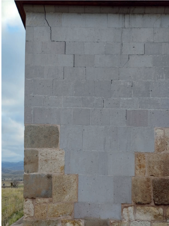
Figure 4. Crack development caused by restoration stones
