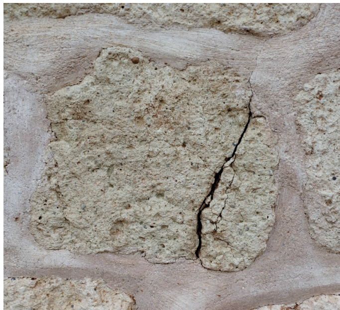
Figure 3. The crack type that develops in the monument
