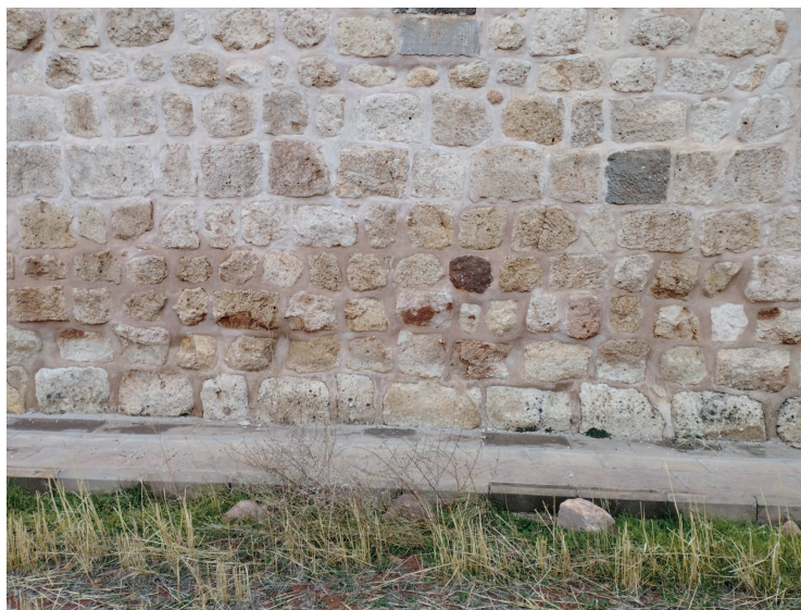
Figure 5. Moist area observed in the structure
