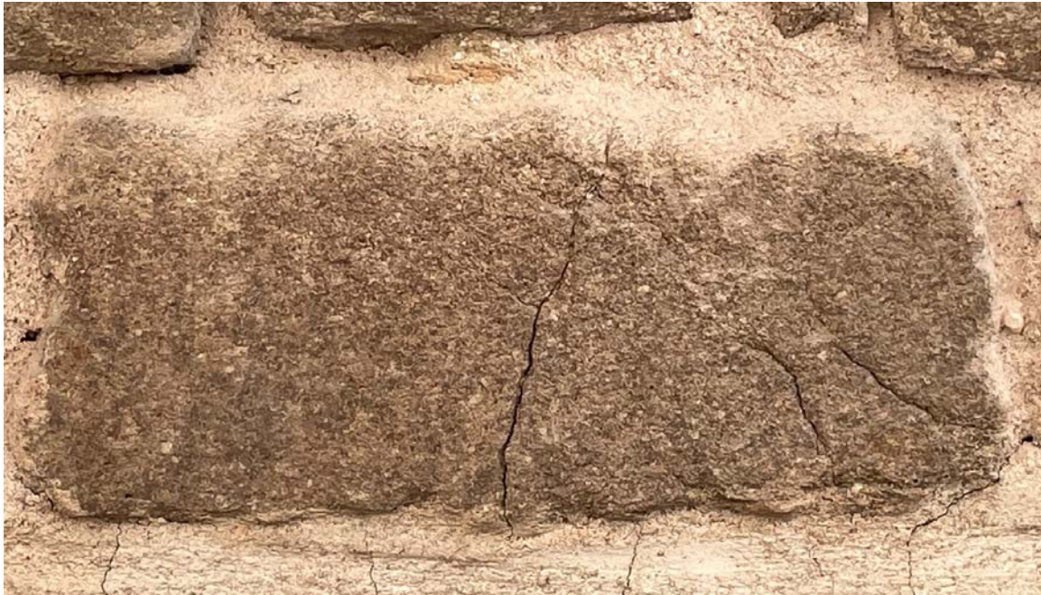
Figure 2. The view of crack anomaly.
