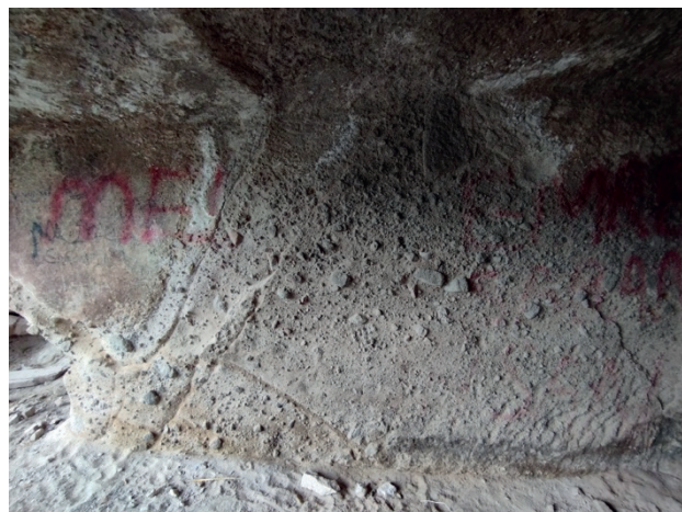
Figure 5. Efflorescence-type deteriorations in the structure
