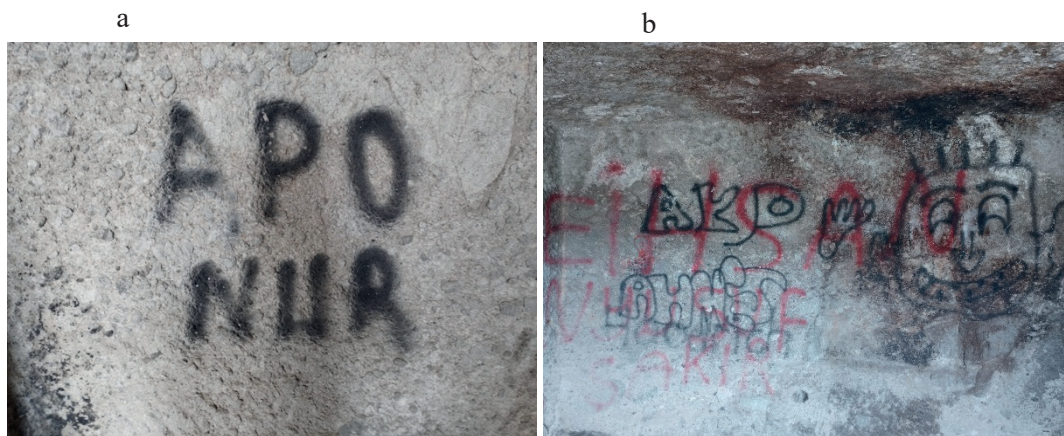
Figure 7. a-b) Graffiti examples on the structure walls
