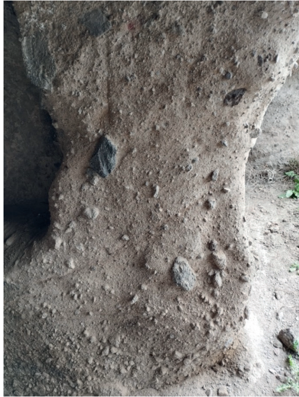
Figure 2. Flaking and differential erosion types observed in Koimesis Tes Panagias Church
