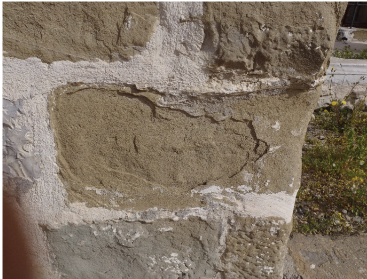
Figure 2. Contour scaling type observed in the monument
