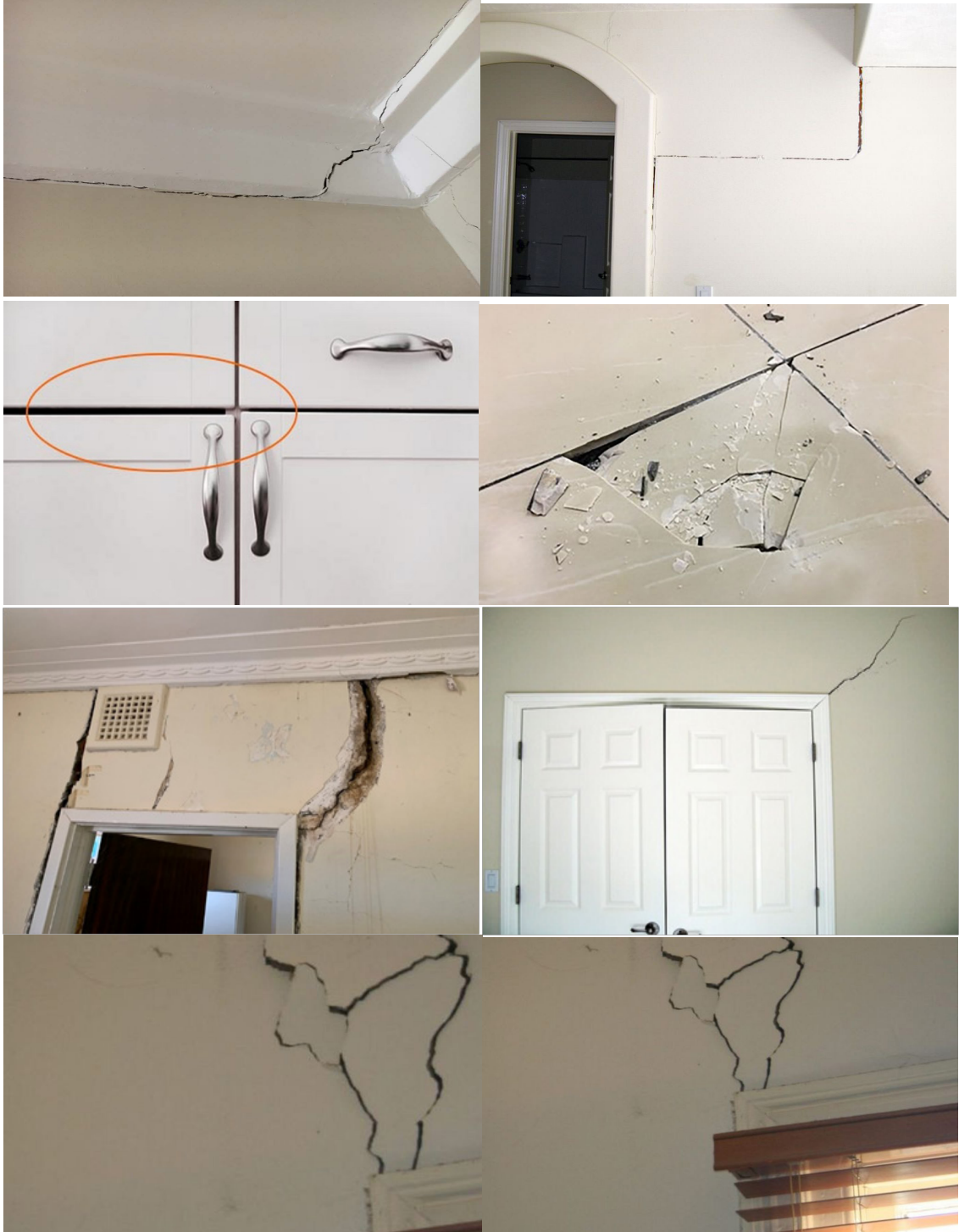
Şekil 68. Obruk belirtileri: Kapı, pencere ve dolaplarda köşelerden ayrılma ve sıkışma, zeminde çatlaklar ( foundationtechs.com/major-sinkhole-signs , 2022; crackedslab.com/blog/do-i-have-signs-of-a-sinkhole-or-foundation-issues , 2023; vipadjusting.com/sinkhole-damage , 2023)
