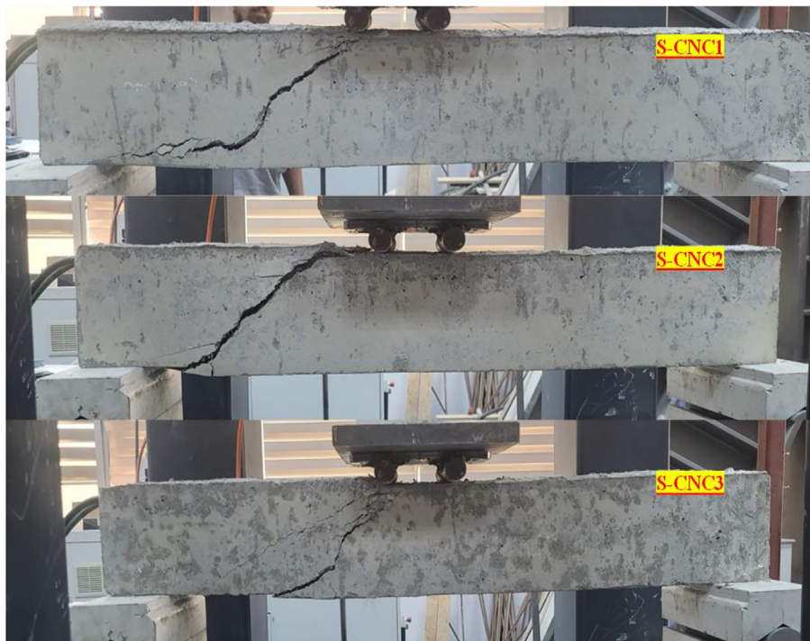
Fig. 7 – Fracture and shear behavior of RCB for S-CNC1, S-CNC2, S-CNC3.
