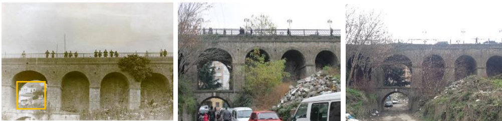
Figure 10. Northern Facade of Tabakhane Bridge; 1920's and Present (URL-3, Bahar Karakaş Archive, 2013; Bahar Karakaş Archive, 2017)
